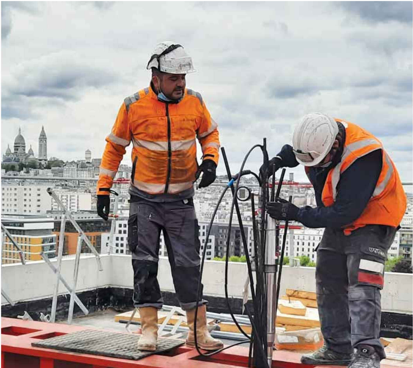
Structural strengthening work underway on the roof of Building 2 of the Chapelle International development in Paris – with the famous Sacré Cœur Basilica in the background.
